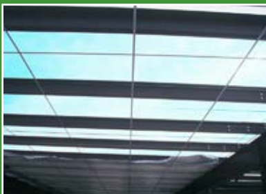
Install the longitudinal and traverse steel strapping to create the strap platform.
