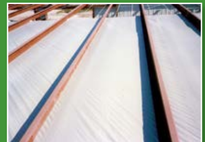
View of fabric liner positioned on strap platform and fastened to the structure.
