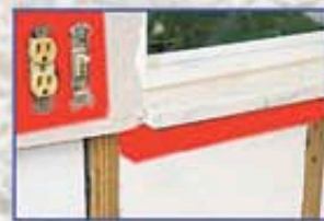
Stop air infiltration through windows, electrical outlets.
